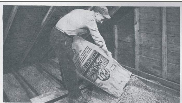
Robert Robson of Dearborn, Michigan, installed Zonolite Vermiculite Insulation in his attic in one afternoon. This insulation will save him many dollars in fuel costs.
