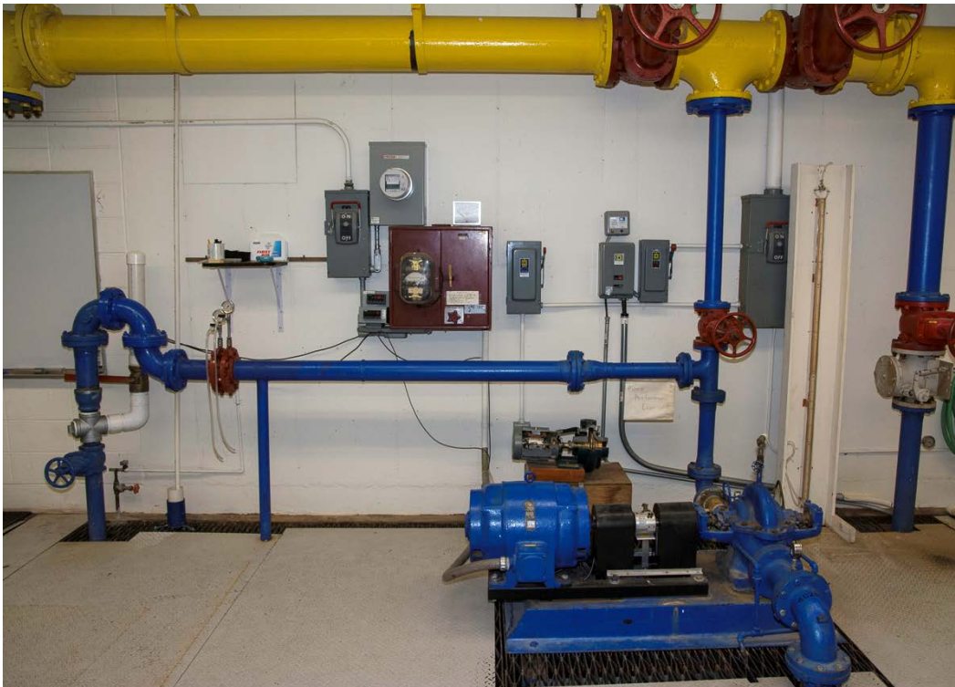
Fig. 9.1: Hydraulics Pumps – Hydraulics and Fluids Lab, 113 Cobleigh Hall
